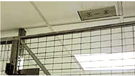
T-DAR DS100 camera in the ceiling above a server cage in a data center.
